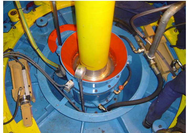
Thordon SXL turbine guide bearing installed at Graus Power Station, Spain
